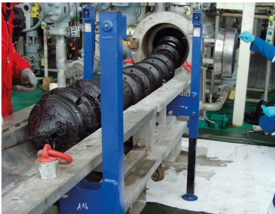
NDT tool being removed from pig receiver
