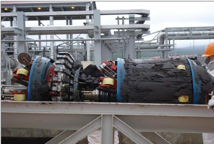
Figure 1: MFL/Geo tool after run in insufficiently cleaned pipeline
