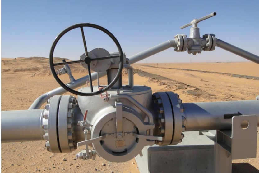
Figure 3: Three-port valve as used for launching cleaning tools
