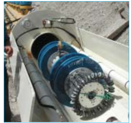
A Weatherford caliper pig awaiting launch on the Blue Stream project.
