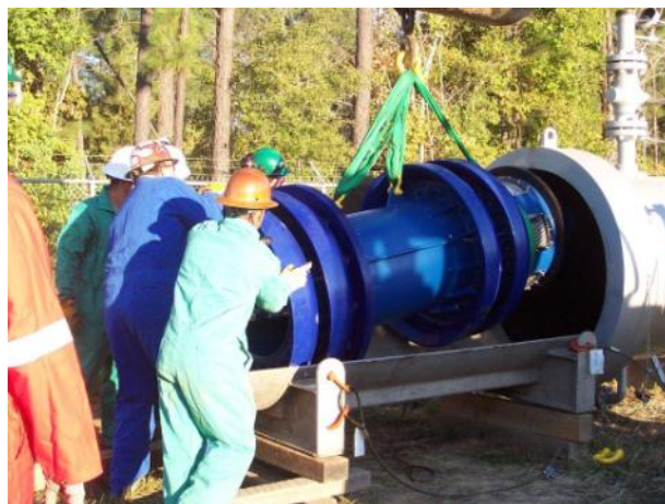
42" Speed Control Pig being launched in high velocity gas pipeline
