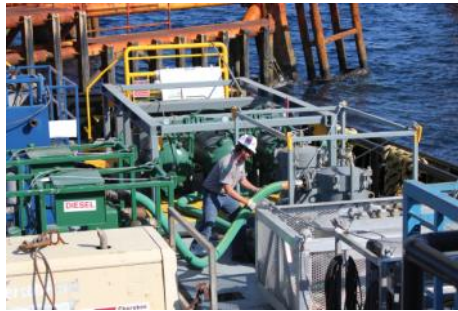
Pipeline flush and abandonment process equipment is set up in the Gulf of Mexico
