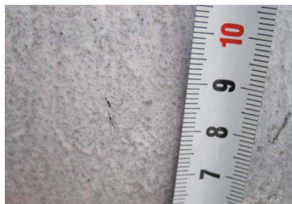
Figure 2: A crack that was found after dig-up work
