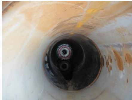
View upstream of the tie-in point showing STATS 36" Tecno Plug™ in the pipeline
