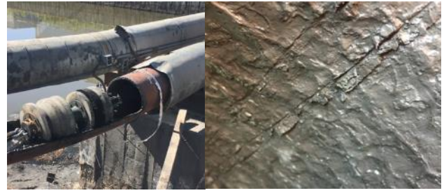
Scraper Pig pull through test & Partial shedding of scale after the pull through test
