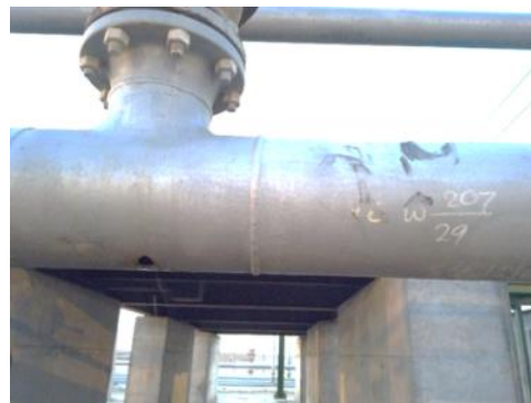
View of tee with through wall defect
