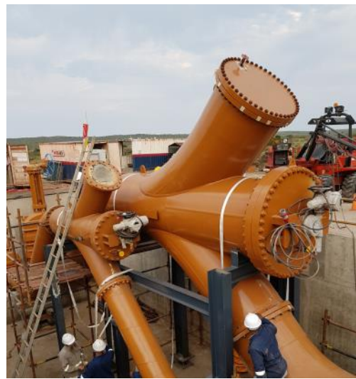
42 inch and 20 inch Pig diverters
