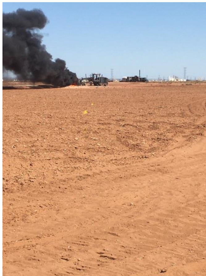
TDW isolates ruptured 14-inch natural gas liquids pipeline
