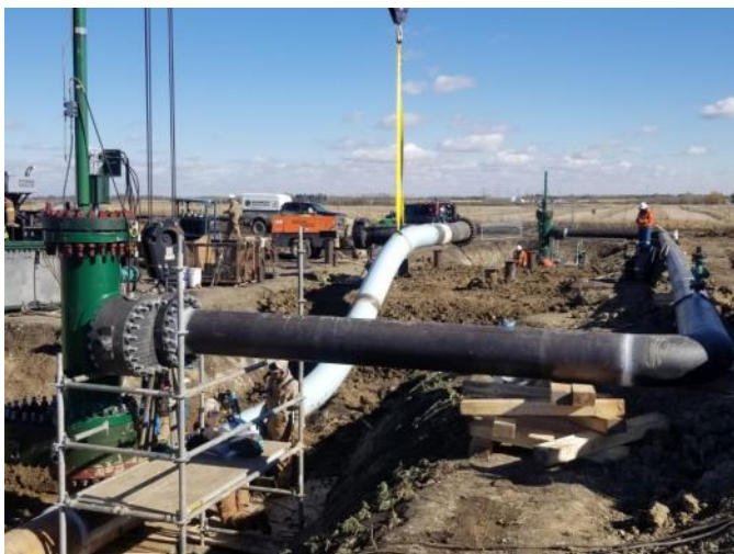
STATS Group's 20 inch BISEP with integrated bypass maintaining production during maintenance and repair
