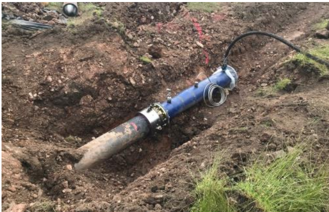
14” x 12”NS temporary pig launcher
