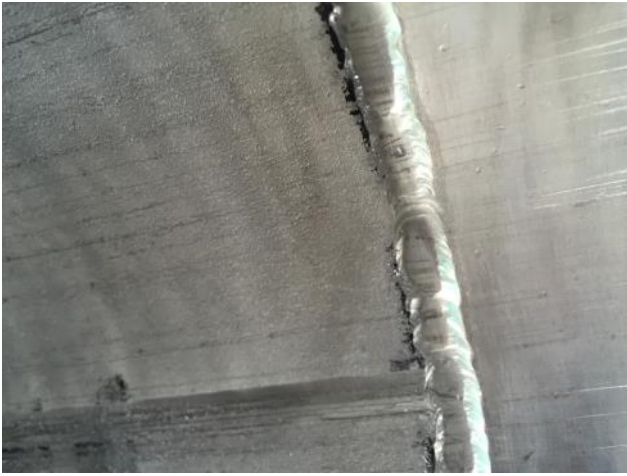
Pipeline inspection after completion of MCT #5 at the start of the line
