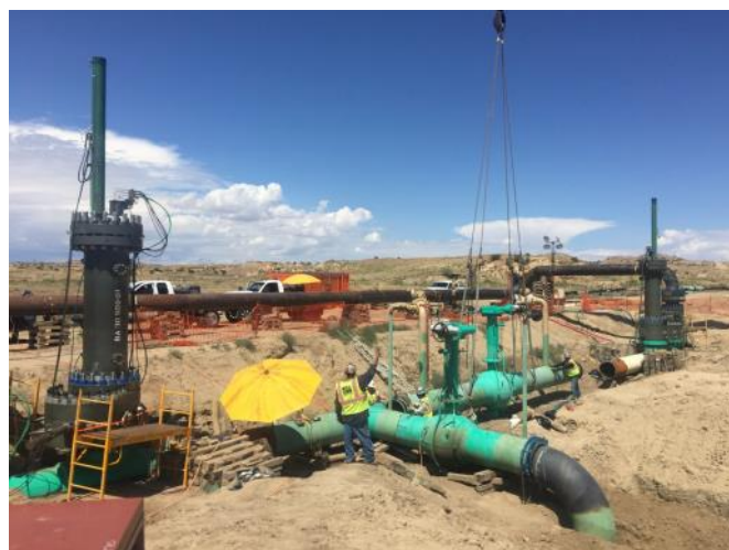
STATS Group 30 inch BISEP isolation CO 2 pipeline
