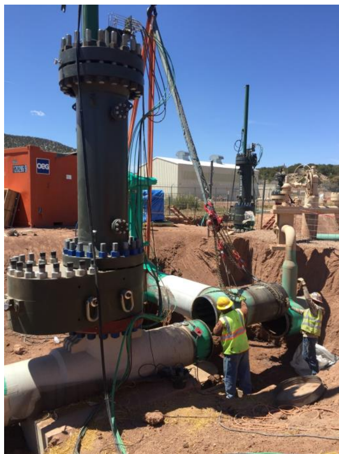
STATS Group 30 inch BISEP isolation CO 2 pipeline
