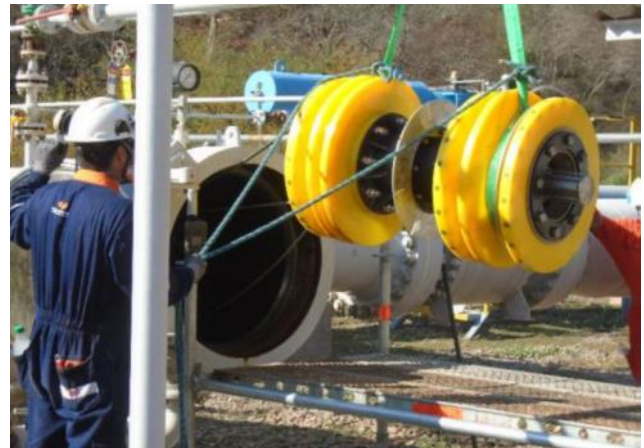
Pig with 28" Gauge Plates being introduced into the throwing trap.
