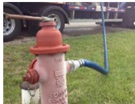
Figure 1. A typical set up for inserting ice into a water main pipeline using a hydrant and two-and-a-half-inch fire hose.
