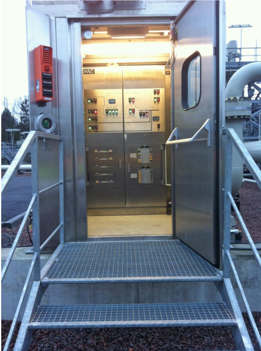
Figure 4: Control Cabinet, integrating mechanical valve interlocking system with electronic safety measures, Nord Stream pigging installation
