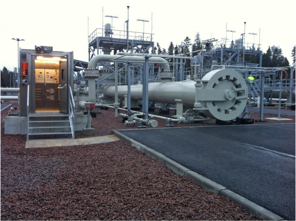
Figure 3: Control cabinet and closure, Nord Stream pigging installation
