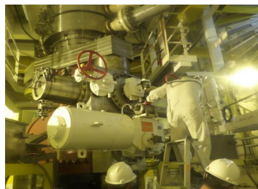
Figure 5: Pigging valve receiver on FPSO.
